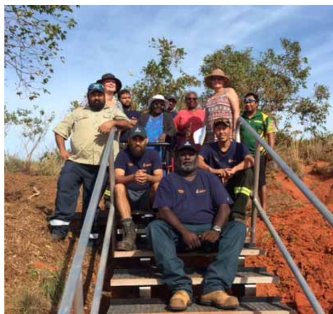
THE NEW STAIRS AT SIMPSON BEACH BUILT BY YAWURU RANGERS AND PARKS AND WILDLIFE
